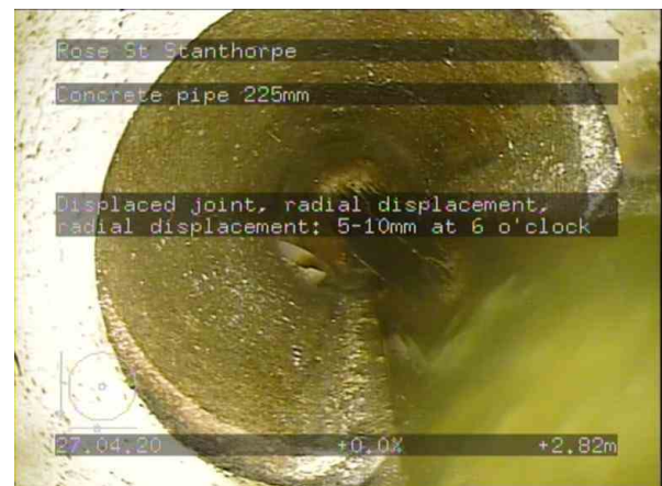
SMH3113 - SMH3645_a0c2278c-0dc2-4ceb-a285-60acb5a37b37_202004 27_082831_449.jpg, 00:03:58, 2.82 Displaced joint, radial displacement, radial displacement: 5-10mm at 6 o'clock
