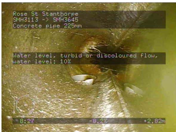
SMH3113 - SMH3645_64d4bb73-3339-45be-b99a-69f05d666b40_202004 27_082812_080.jpg, 00:03:47, 2.82 Water level, turbid or discoloured flow, water level: 10%
