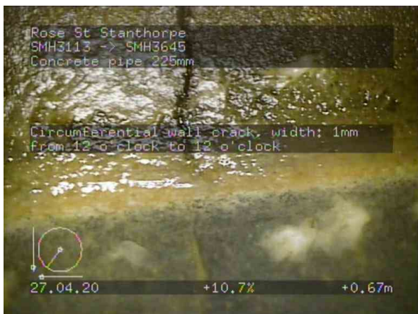
SMH3113 - SMH3645_5f7be426-3515-463c-ae9e-3a50f1e30f52_2020042 7_082347_098.jpg, 00:01:30, 0.67 Circumferential wall crack, width: 1mm from 12 o'clock to 12 o'clock
