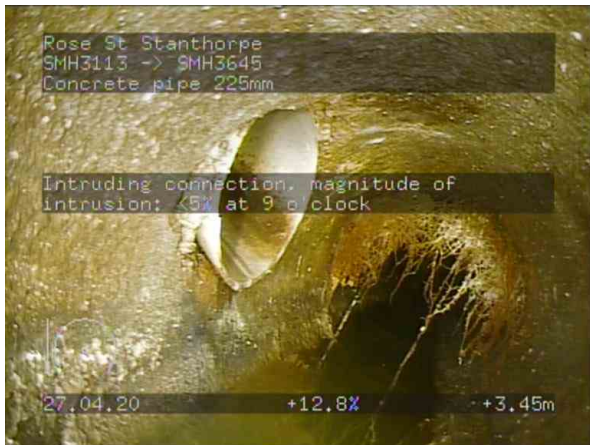
SMH3113 - SMH3645_8e5c4093-05a4-4d6e-84a7-065e190622e5_20200427_082926_472.jpg, 00:04:27, 3.45 Intruding connection, magnitude of intrusion: <5% at 9 o'clock
