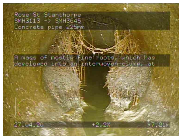
SMH3113 - SMH3645_820c074b-1e0f-47aa-8af1-7b3a16a7871d_20200427_083201_671.jpg, 00:06:30, 7.21 A mass of mostly fine roots, which has developed into an interwoven clump, at joint, Obstruction: 21-50% from 12 o'clock to 12 o'clock
