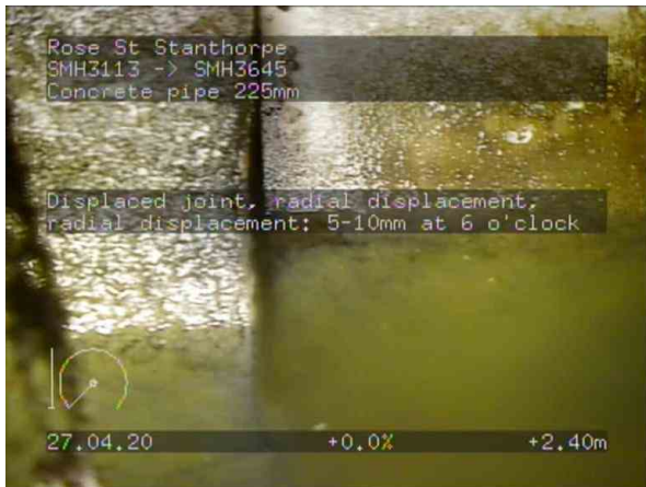
SMH3113 - SMH3645_665492aa-3c9e-42dd-8f26-2fa9405c0485_202004 27_082523_289.jpg, 00:02:44, 2.40 Displaced joint, radial displacement, radial displacement: 5-10mm at 6 o'clock
