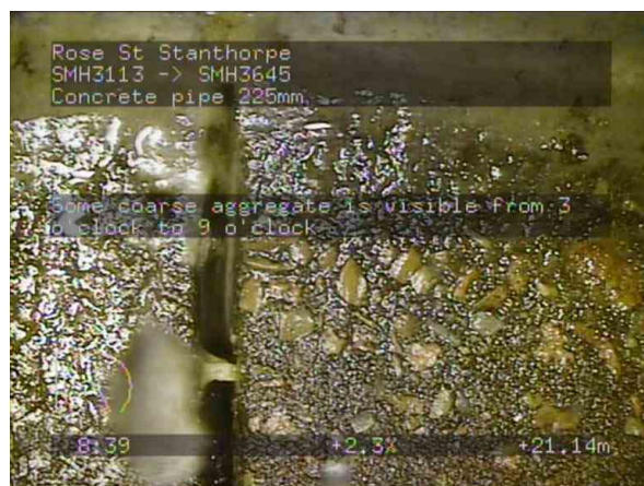
SMH3113 - SMH3645_8e26d9a6-f200-4a67-ab1a-63c0deb0f079_20200427_084013_661.jpg, 00:12:39, 21.14 Some coarse aggregate is visible from 3 o'clock to 9 o'clock
