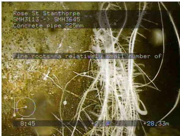
SMH3113 - SMH3645_8aa7db36-cc52-4599-a904-ffbc53c0579c_20200427_084538_119.jpg, 00:16:29, 28.33 Fine roots--a relatively small number of flexible minor roots, Obstruction: <5% from 7 o'clock to 12 o'clock
