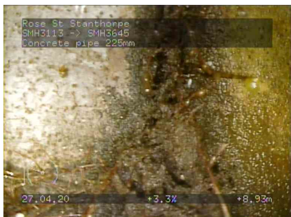
SMH3113 - SMH3645_ac99604e-5eb2-4022-bd8a-2951b35ec24c_20200427_083251_180.jpg, 00:07:07, 8.93 Fine roots--a relatively small number of flexible minor roots, Obstruction: <5% from 12 o'clock to 12 o'clock
