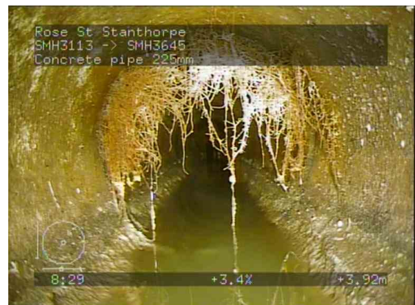
SMH3113 - SMH3645_2c652f55-5860-43fa-a582-48ae9676d206_20200427_083024_702.jpg, 00:04:57, 3.92 A mass of mostly fine roots, which has developed into an interwoven clump, Obstruction: 5-20% from 8 o'clock to 4 o'clock
