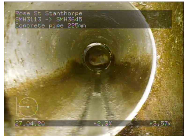
SMH3113 - SMH3645_6a1202b8-fdfb-4994-adcd-5b474aa18ad6_20200427_082939_776.jpg, 00:04:27, 3.45 Intruding connection, magnitude of intrusion: <5% at 9 o'clock
