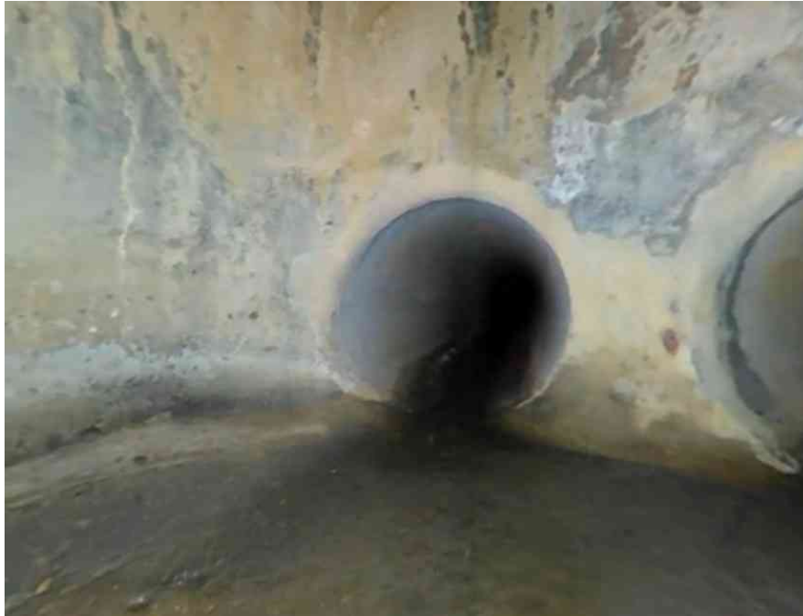
3, 00:00:11, 1.20 A conduit connecting to the maintenance structure, circular, incoming., Ht/Dia # 375mm at 4 o'clock
