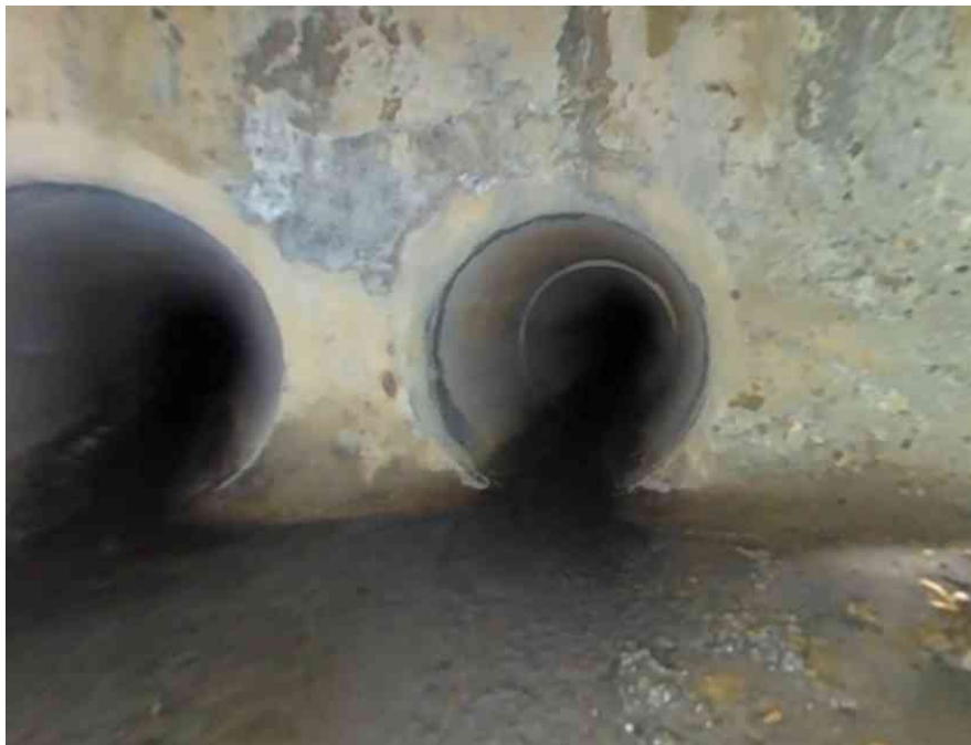
4, 00:00:11, 1.20 A conduit connecting to the maintenance structure, circular, incoming., Ht/Dia # 375mm at 6 o'clock
