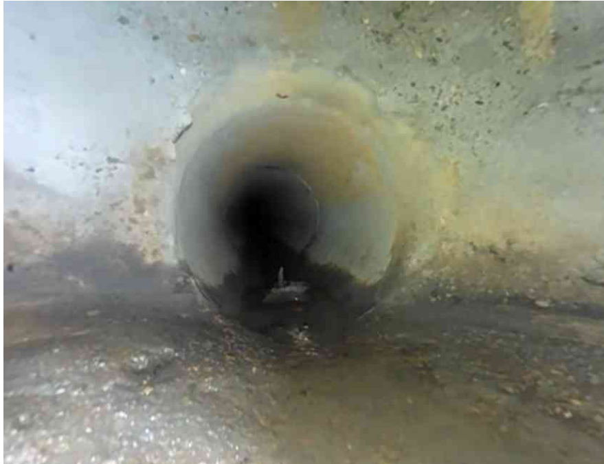
5, 00:00:11, 1.20 A conduit connecting to the maintenance structure, circular, outgoing., Ht/Dia # 375mm at 12 o'clock
